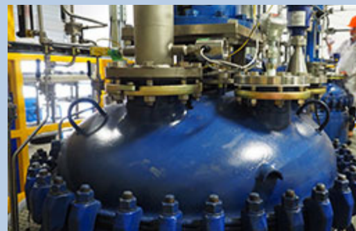
Figure 1: Demonstration Pilot Plant
