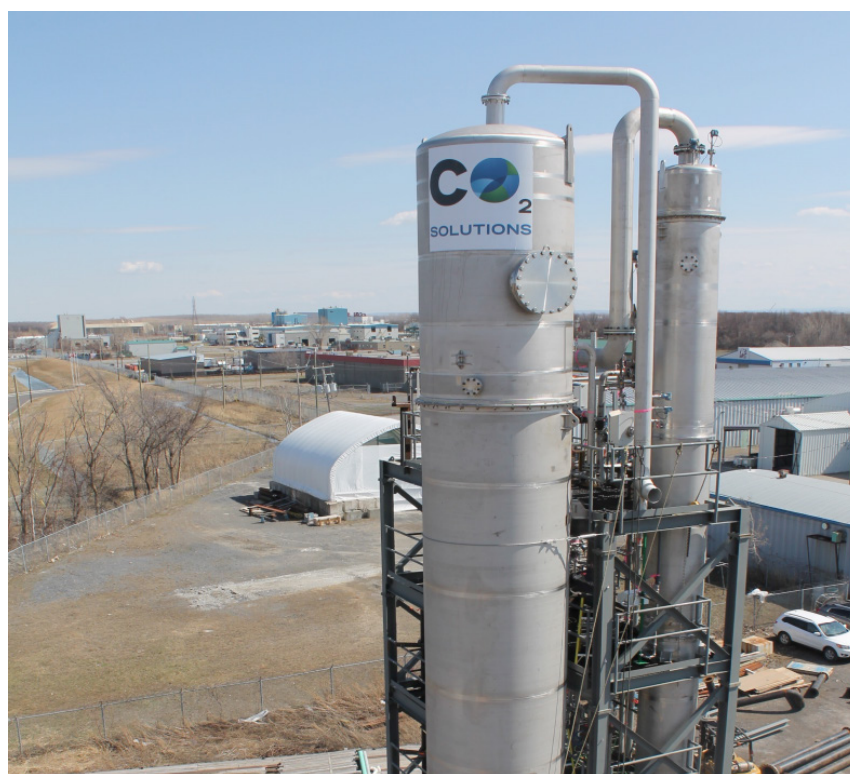
Figure 4: CO 2 Solutions Carbon Capture Unit
